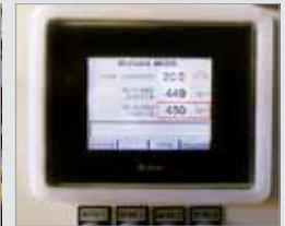
6 Control panel display
